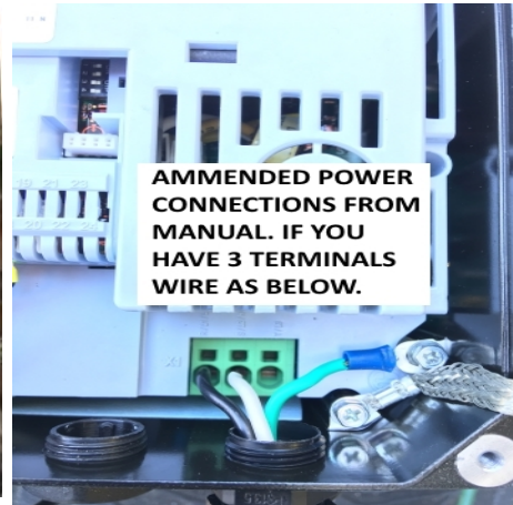
3 TERMINAL DRIVE POWER HOOK UP
